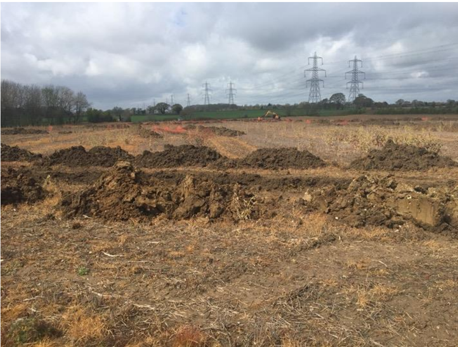
Annex 5: Open Trench adjacent to Footpath 6 on 12 May 2021 – note dead vegetation
